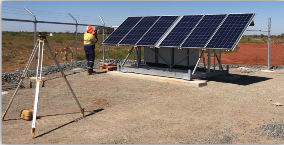
Source : SPS DC power system Wodgina
