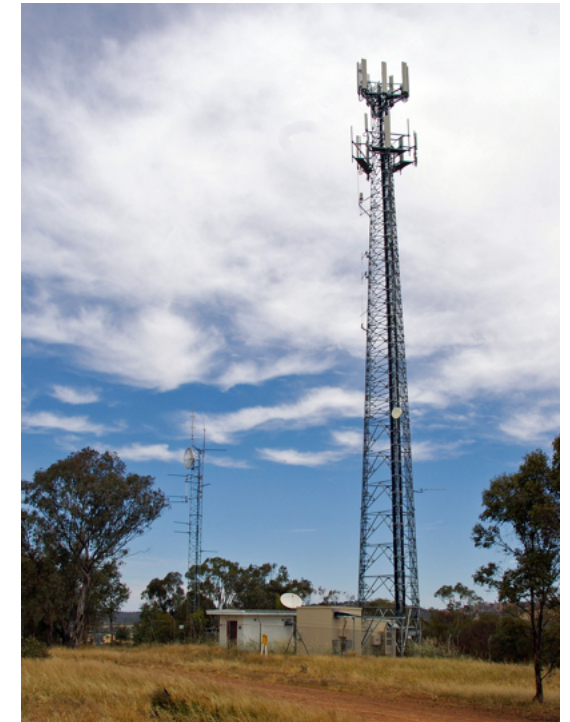
Future Engineering & Communication Telstra tower
