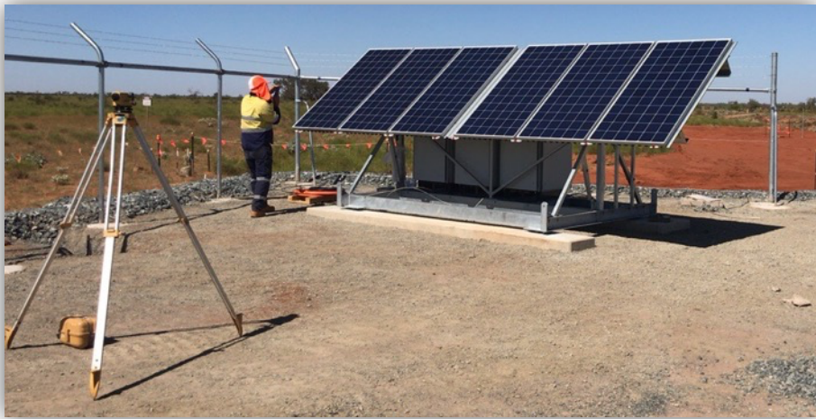
Source : SPS DC power system Wodgina
