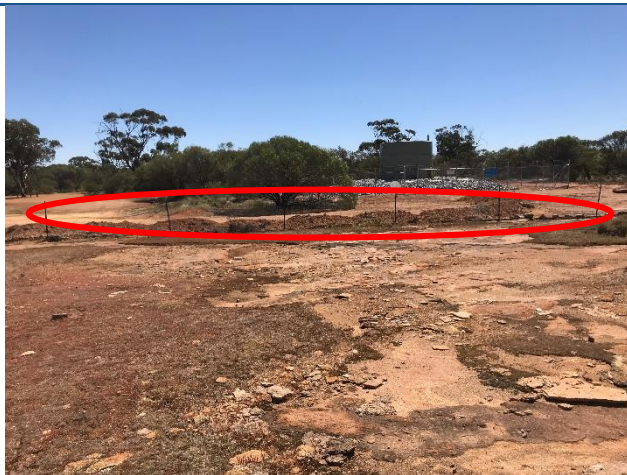
View of existing wire and steel fence separating the rock area from the car park/camping area. The fence is somewhat dilapidated.
