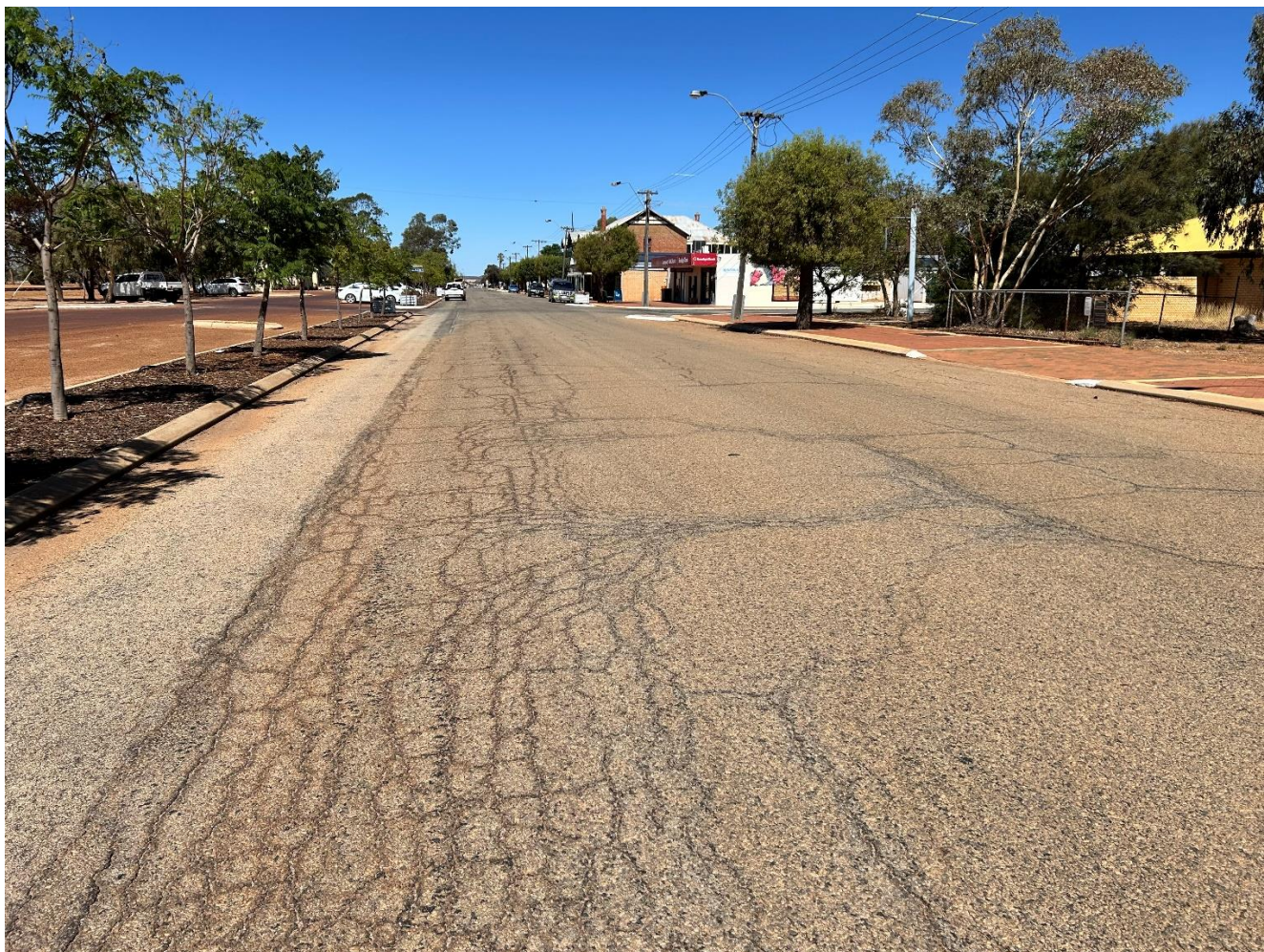
Above Shadbolt Street 2024 – note severe surface cracking
