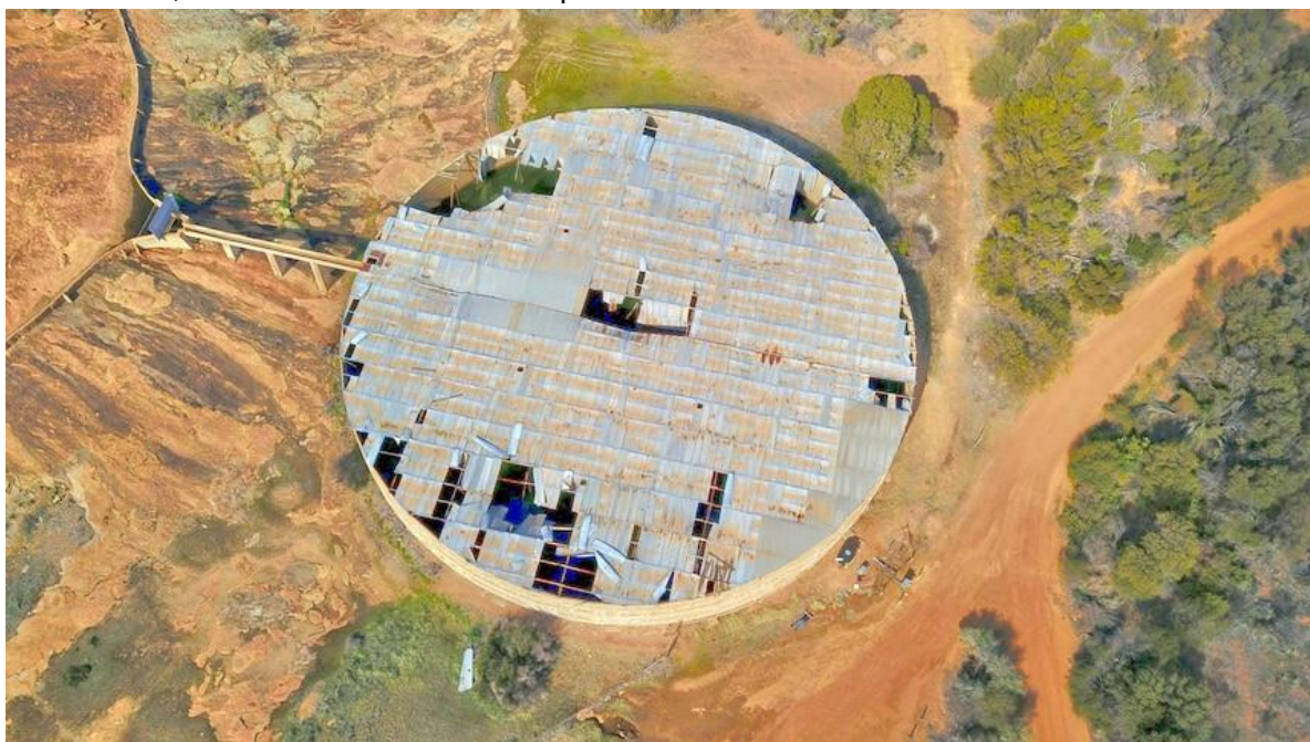
Above: Beringbooding Roof tank November 2020.
